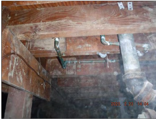
13.0 WATER SUPPLY PIPING (EXPOSED) (Picture 1)
