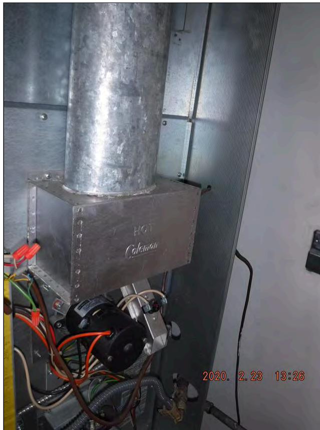
12.0 HEATING UNIT (Picture 1)
