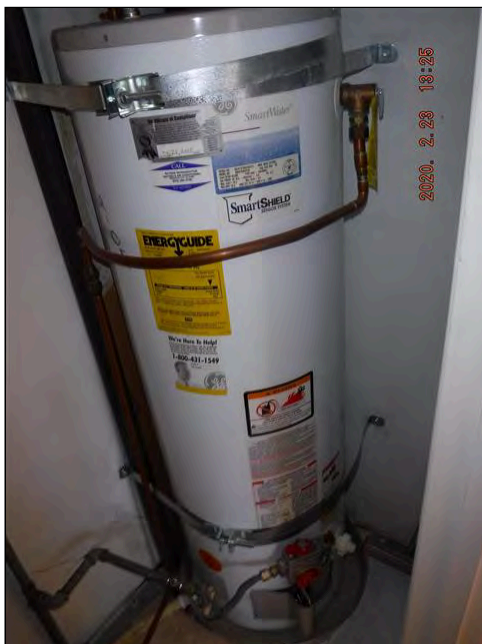
14.0 WATER HEATER (Picture 1)
