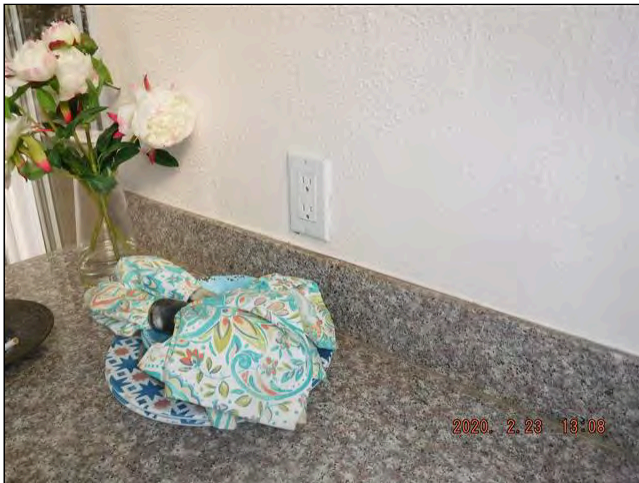
2.4 ELECTRIC / GFCI(S) (Picture 1)
