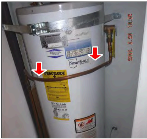
14.4(1) SAFETY VALVE PROVISIONS (Picture 1)
