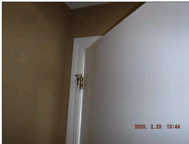
4.7 HOUSE / SERVICE DOOR(S) (Picture 1)
