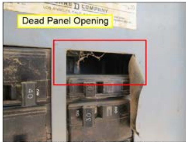
9.2 DISTRIBUTION PANEL Picture 1
