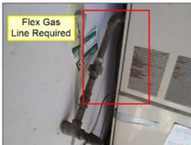
11.2.D GAS / FUEL LINES AT UNIT Picture 1
