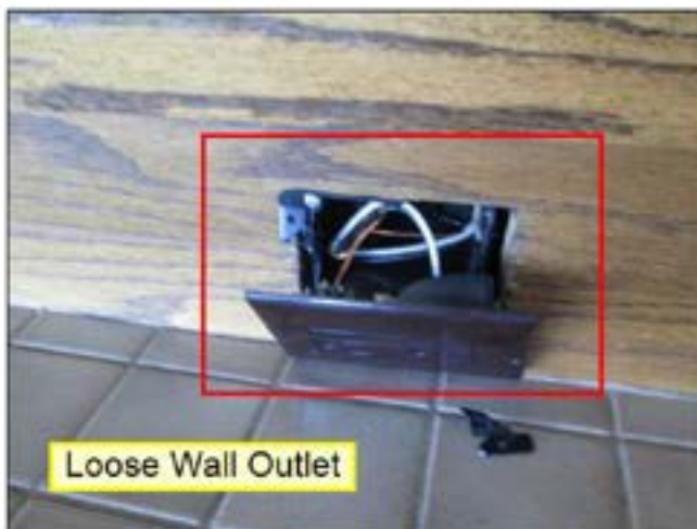
7.3.A ELECTRIC / GFCI Picture 1
