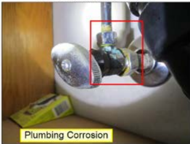
12.0 WATER PIPING Picture 3
