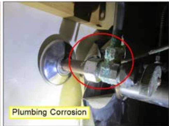
12.0 WATER PIPING Picture 2
