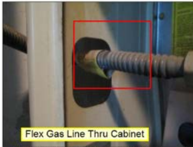
11.2.B GAS / FUEL LINES AT UNIT Picture 1
