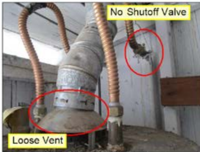
13.0.B WATER HEATER Picture 3
