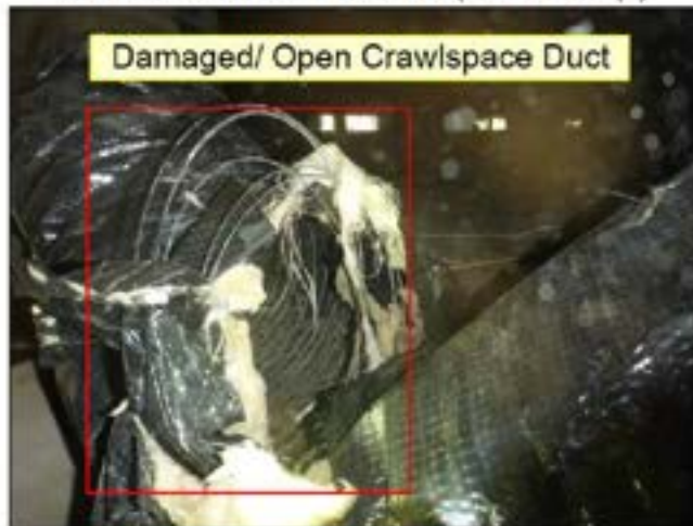
9.5 DISTRIBUTION SYSTEM (See Picture(s))
