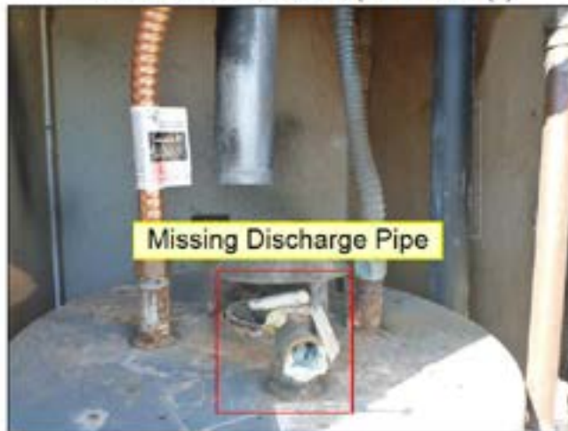
11.3 SAFETY VALVE PROVISIONS (See Picture(s))
