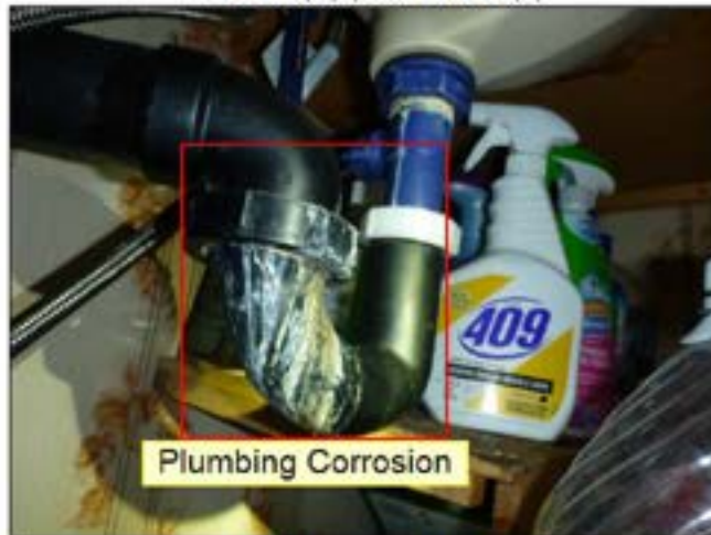
4.0 SINK(S) (See Picture(s))
