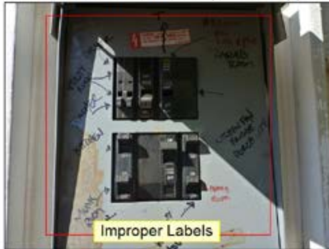
8.0 DISTRIBUTION PANEL (See Picture(s))
