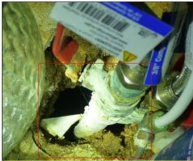
Heavy Corrosion/ Holes In Sub-Floor
