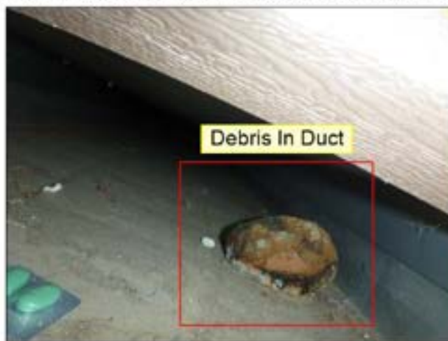
9.5 DISTRIBUTION SYSTEM (See Picture(s))
