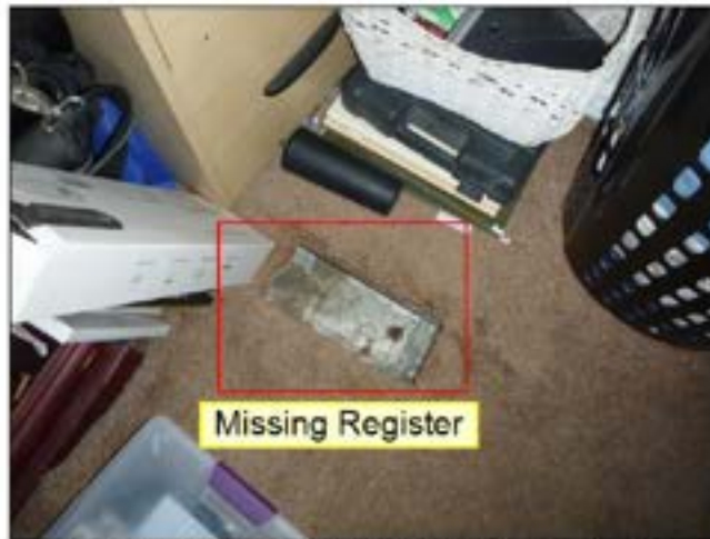
9.5 DISTRIBUTION SYSTEM (See Picture(s))
