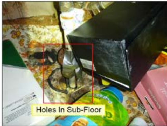
4.0 SINK(S) (See Picture(s))
