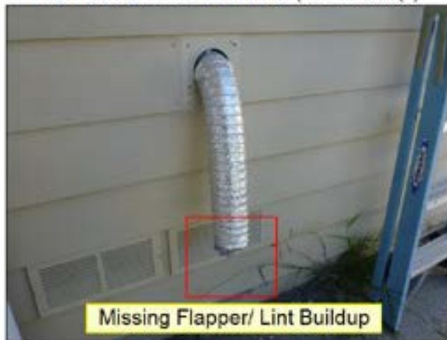
10.3 Dryer Vent (See Picture(s))
