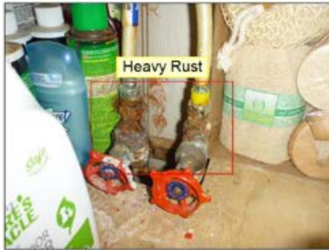
4.0 SINK(S) (See Picture(s))
