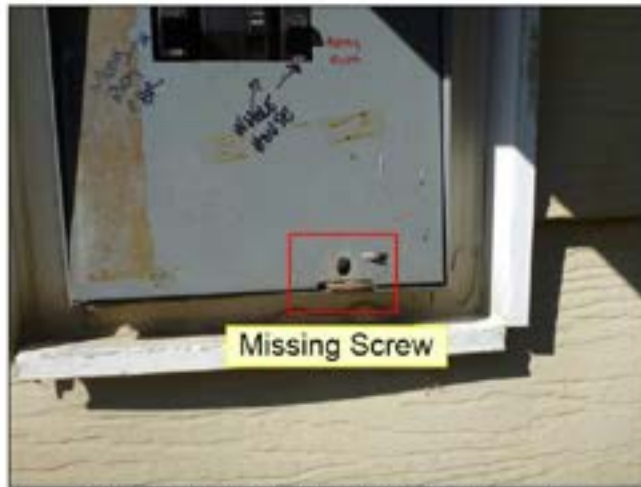
8.0 DISTRIBUTION PANEL (See Picture(s))
