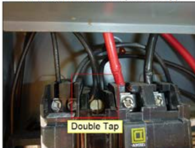
8.0 DISTRIBUTION PANEL (See Picture(s))
