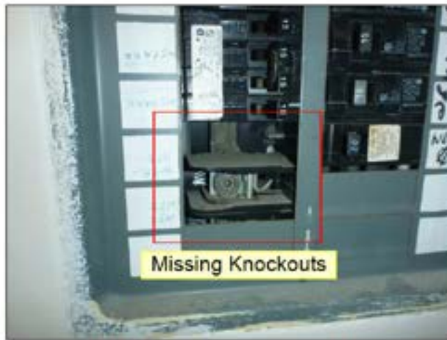
6.4 SUBPANEL(S) (See Picture(s))
