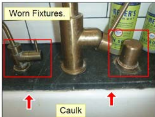
4.0.B PLUMBING / SINK (See Picture(s))
