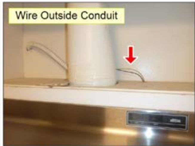
4.3.J ELECTRIC / GFCI (See Picture(s))
