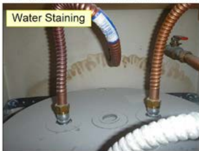
9.0.K WATER HEATER (See Picture(s))
