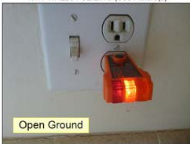
4.3.V(2) ELECTRIC / GFCI (See Picture(s))
