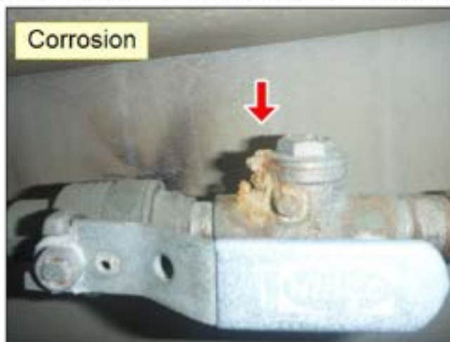
9.0.B WATER HEATER (See Picture(s))
