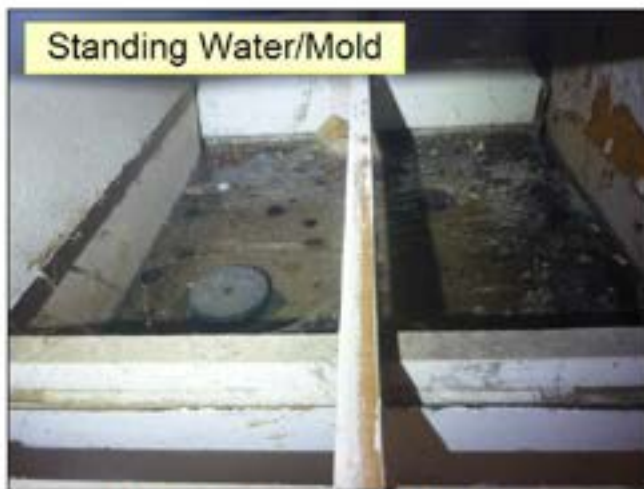
4.0.C PLUMBING / SINK (See Picture(s))
