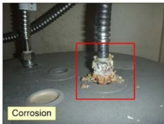
9.0.M WATER HEATER (See Picture(s))
