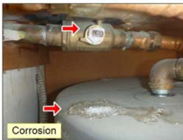
9.0.S WATER HEATER (See Picture(s))
