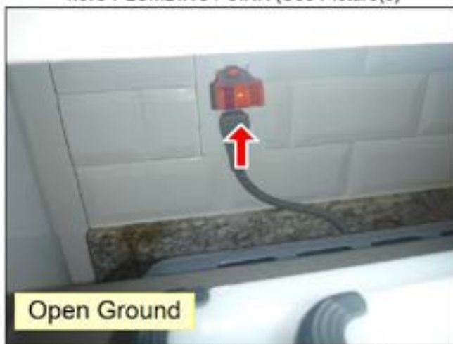
4.2.C ELECTRIC / GFCI (See Picture(s))
