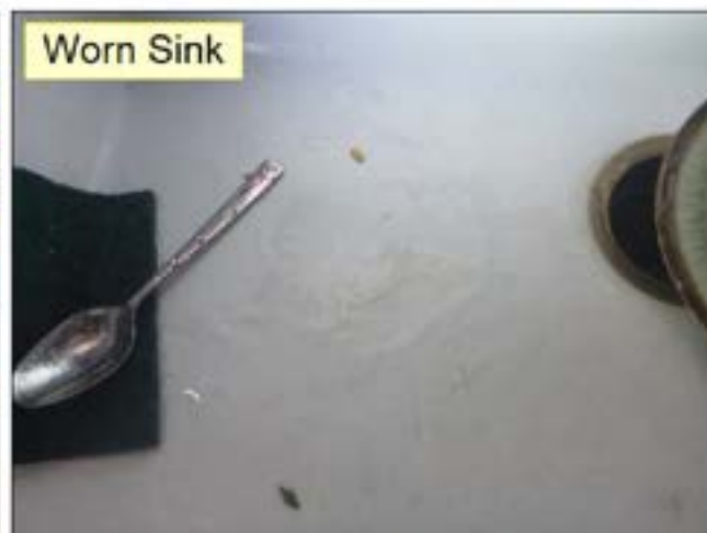
4.0.B PLUMBING / SINK (See Picture(s))
