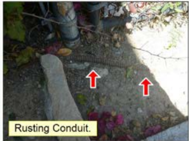
1.6 ELECTRIC / GFCI (See Picture(s))
