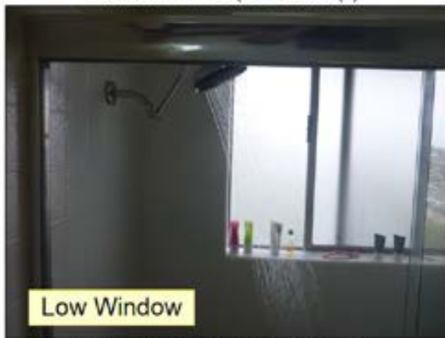
3.5.K VENTILATION (See Picture(s))
