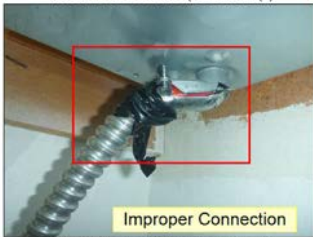
4.3.J ELECTRIC / GFCI (See Picture(s))
