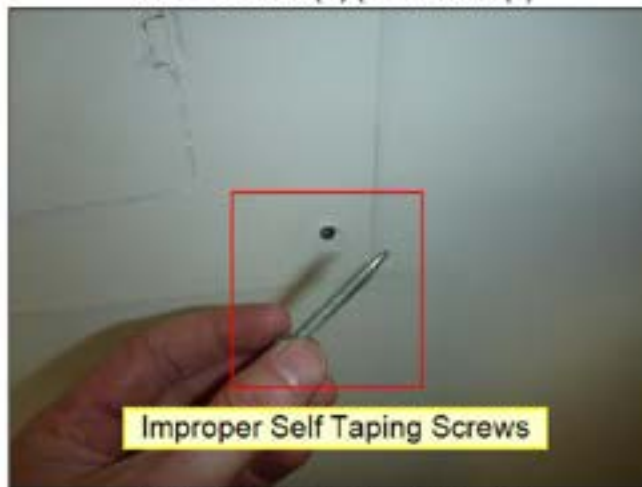
6.4 SUBPANEL(S) (See Picture(s))
