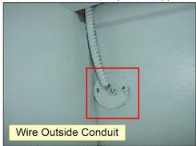
4.3.J ELECTRIC / GFCI (See Picture(s))
