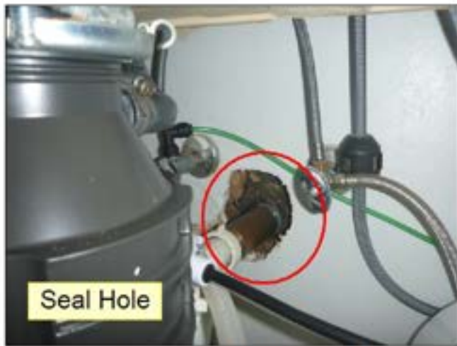
4.1.J WALLS / CEILING (See Picture(s))
