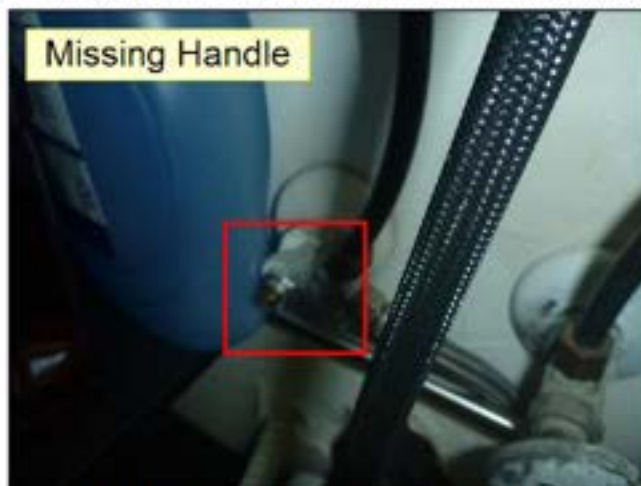
4.0.Z PLUMBING / SINK (See Picture(s))
