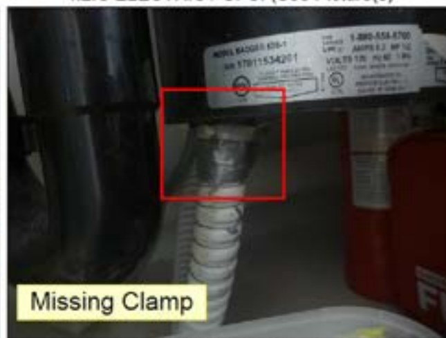
4.2.C ELECTRIC / GFCI (See Picture(s))
