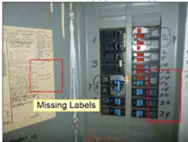
6.4 SUBPANEL(S) (See Picture(s))
