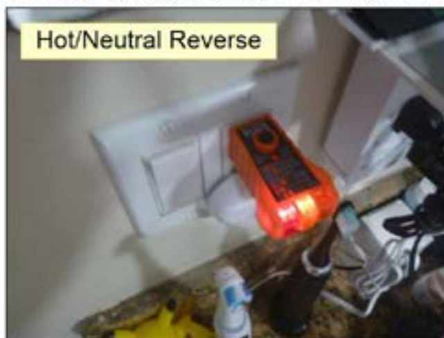
3.3.Q ELECTRIC / GFCI (See Picture(s))
