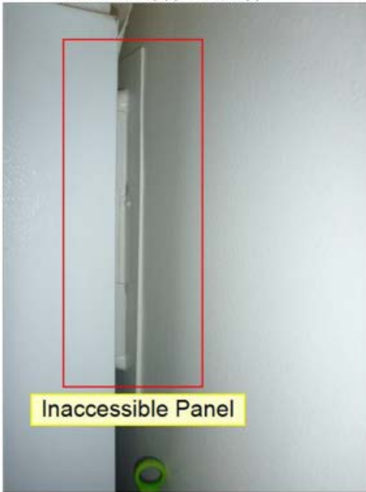
6.4 SUBPANEL(S) (See Picture(s))
