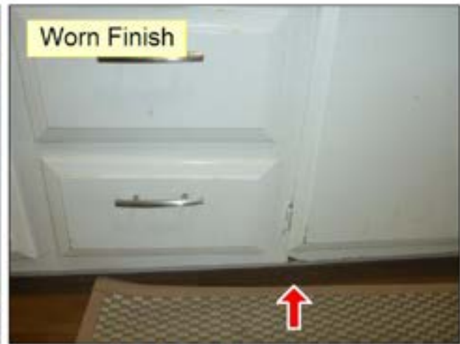
4.8.M CABINETS (See Picture(s))
