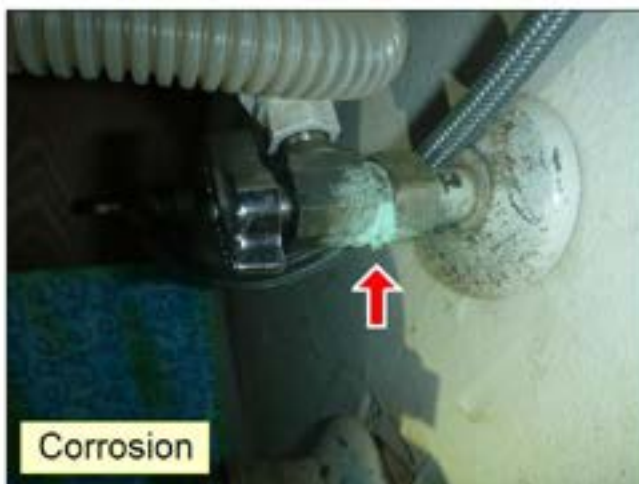
4.0.P PLUMBING / SINK (See Picture(s))
