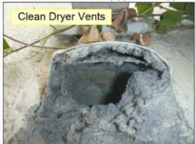
8.6 Dryer Vent (See Picture(s))
