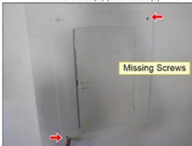
6.4 SUBPANEL(S) (See Picture(s))
