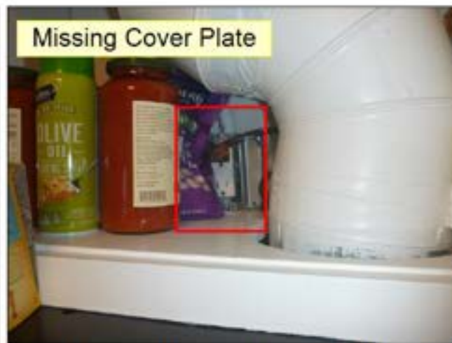
4.2.C ELECTRIC / GFCI (See Picture(s))
