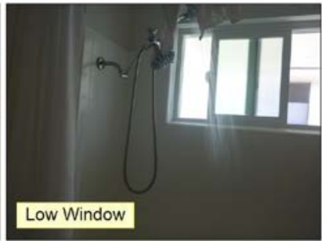
3.4.R VENTILATION (See Picture(s))
