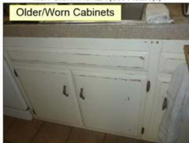
4.7.Y CABINETS (See Picture(s))
