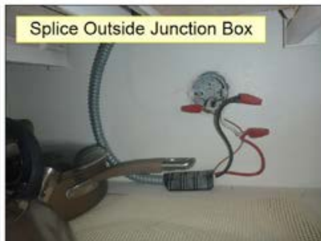
4.2.E ELECTRIC / GFCI (See Picture(s))
