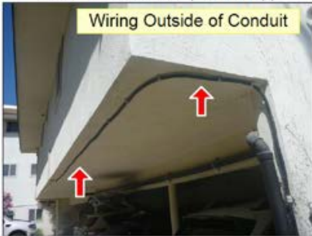
1.6 ELECTRIC / GFCI (See Picture(s))
