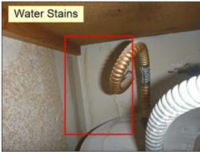
9.0.F WATER HEATER (See Picture(s))
