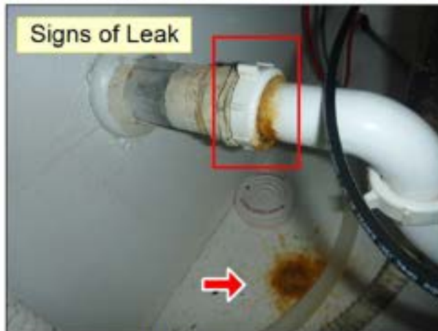
4.0.W PLUMBING / SINK (See Picture(s))
